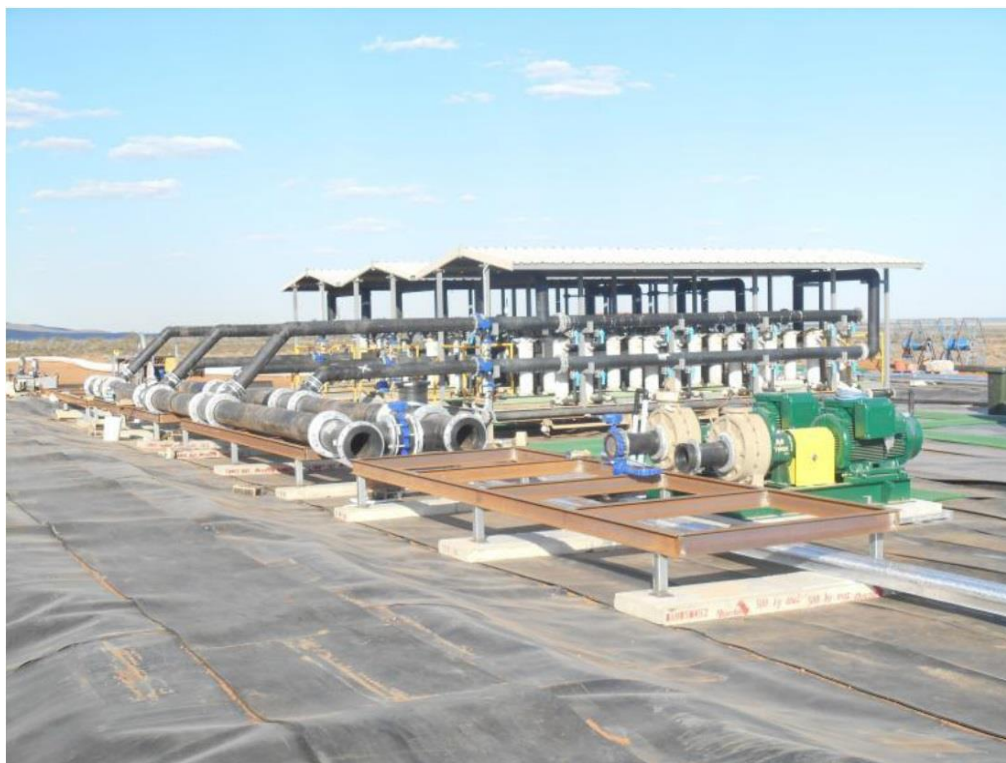
Figure 5: Injection booster and filter skids
