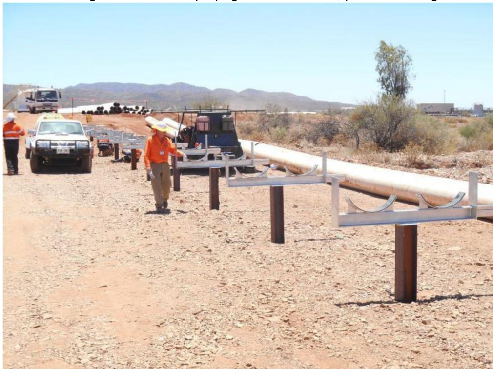
Figure 4: Creek crossing trunkline supports – Pannikan Creek
