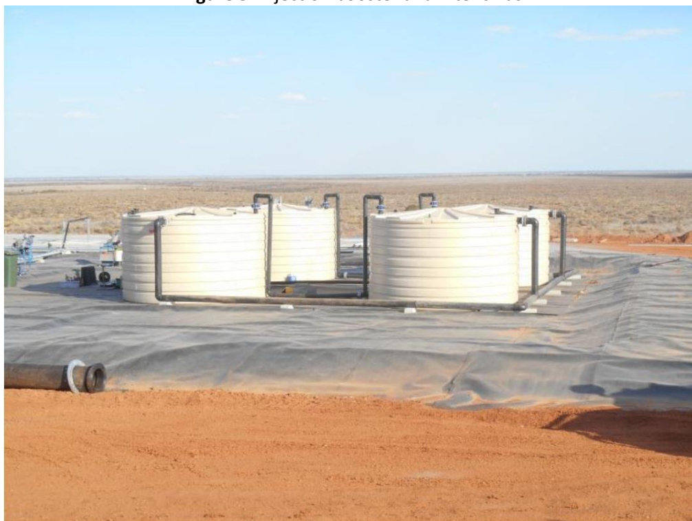
Figure 6: Ferric holding tanks and bund
