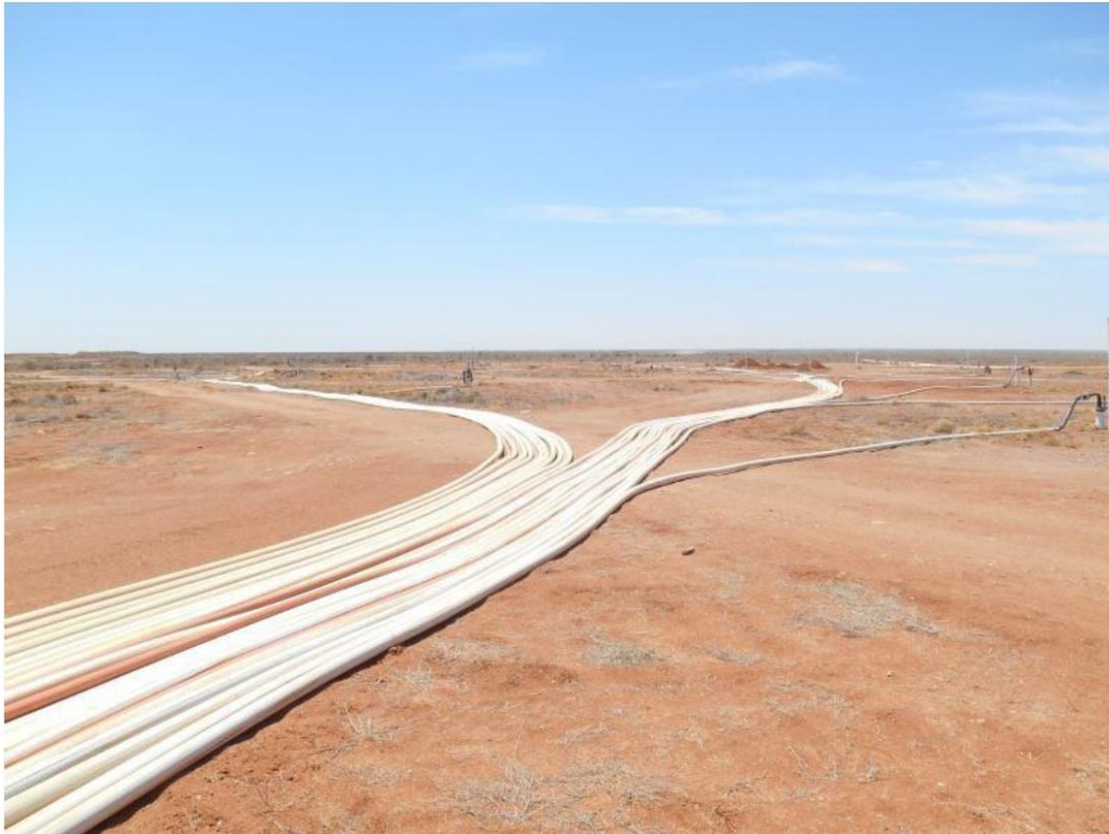
Figure 1: Installation of pipework (“lateral spiders”) from the wellhouses to the FME wellfields
